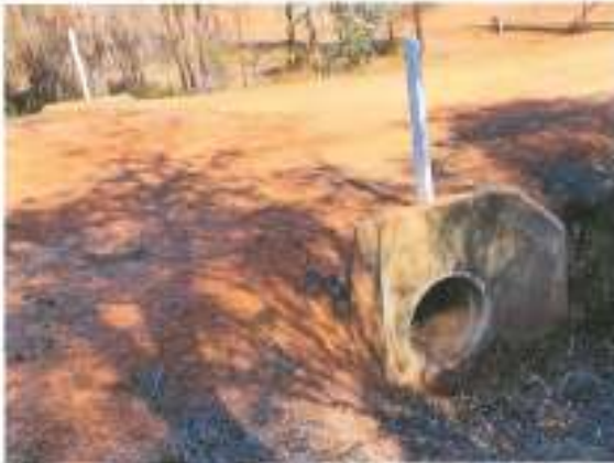
Western end of the culvert showing the concrete headwall over the end of the pipe and the white marker post
