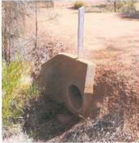
Eastern end of the culvert showing the concrete headwall and compacted gravel
