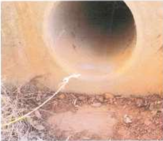
Eastern end of the culvert showing the concrete footing at the base of the pipe
